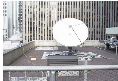
Figure 1 Domestic Ku-band Earth Station Located on Urban Rooftop
